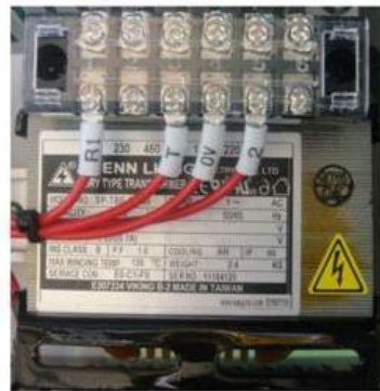
◆ Transformer for 460V.
