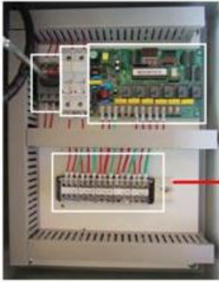
Main Electrical Components for SDC-15-16 Pulse Control Box
