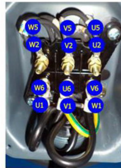
◆ Connecting to motor.
