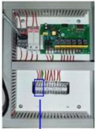
◆ Connecting to the pulse control box.
