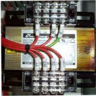
◆ Transformer for 460V.
