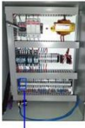
◆ Connecting to the RM-6000 control box.
