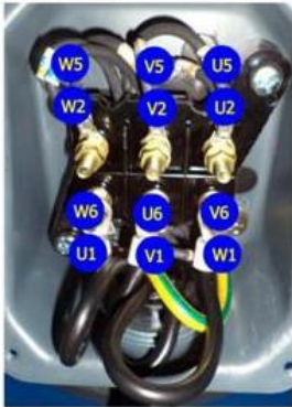
◆ Connecting to motor.
