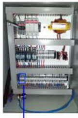
◆ Connecting to the RM-6000 control box.
