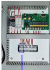
◆ Connecting to the pulse control box.
