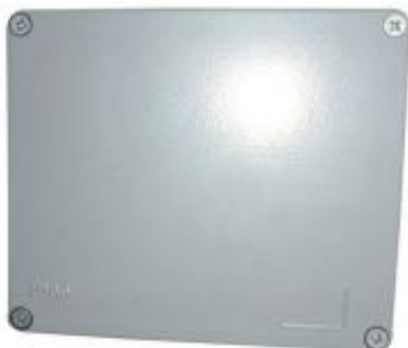
◆ Electrical junction box.
