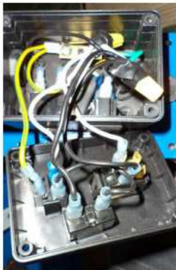
The wiring of light switch
