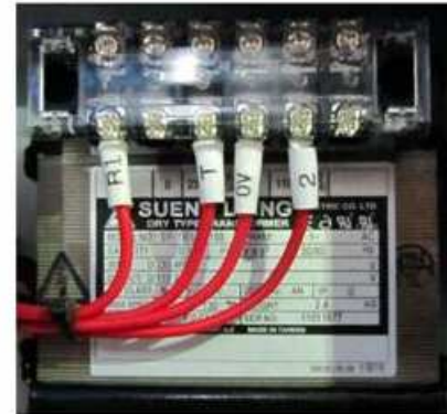
◆ Transformer for 460V.
