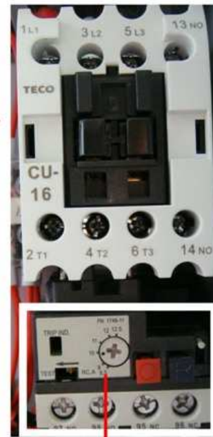
◆ Contactor and thermal relay. (7.5HP-460V)
