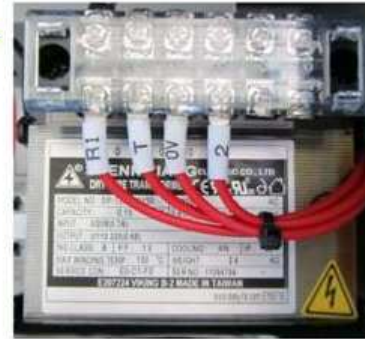
◆ Transformer for 208V.
