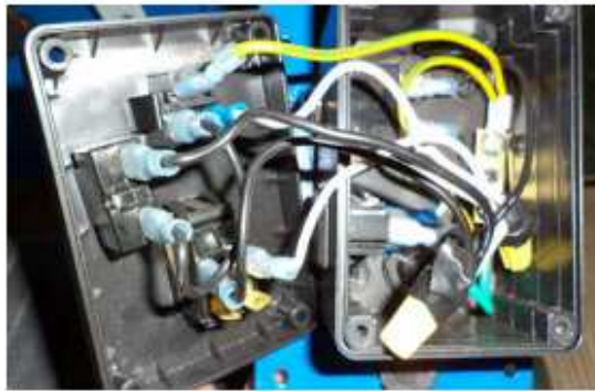
The wiring of light switch
