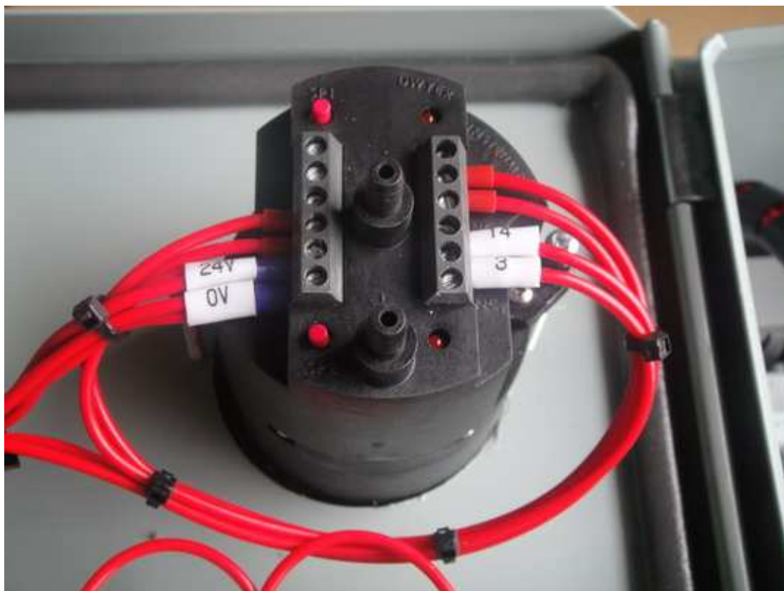
4. gauge connections close-up.
