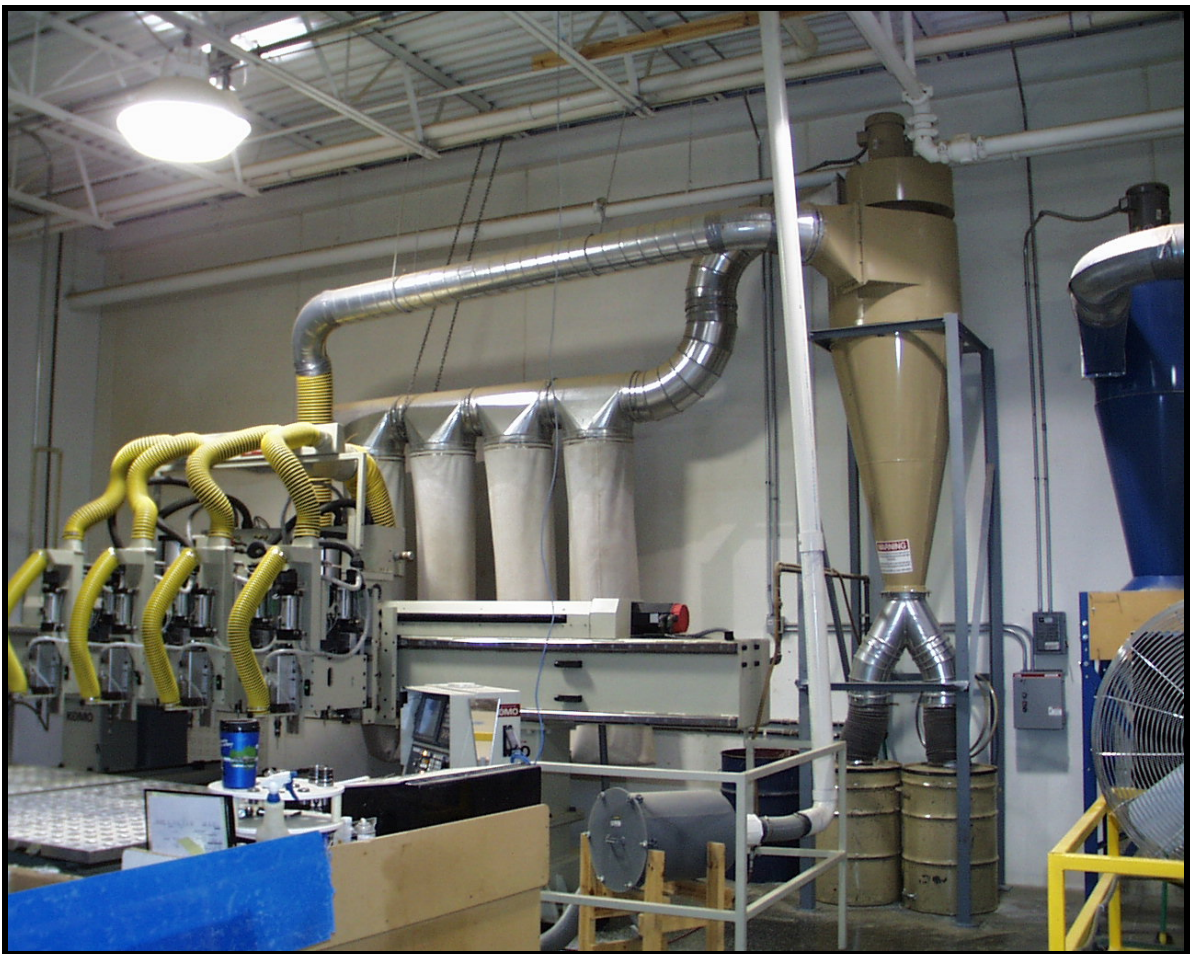
Cyclone with CSP20-4 plenum after-filter
