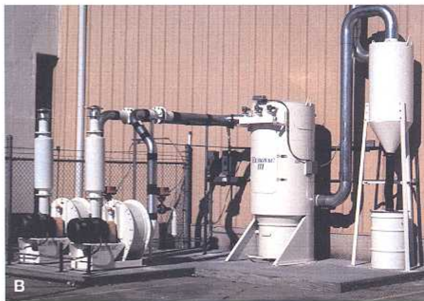
A Eurovac III 20 HP Centrifugal Multi-Stage Pump and 30' Separator.
