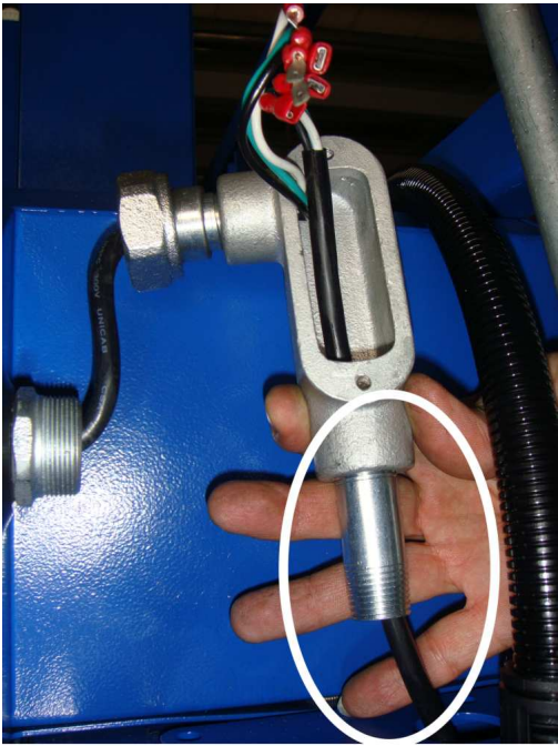
◆ Then reach the cable of the light switch through the tube into the steel adapter box.
